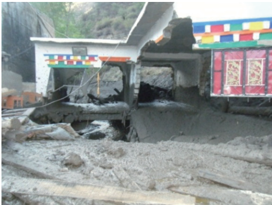
图 4 被泥石流冲毁的房屋 Fig. 4 Site photo of the ruined houses destroyed by debris flows
