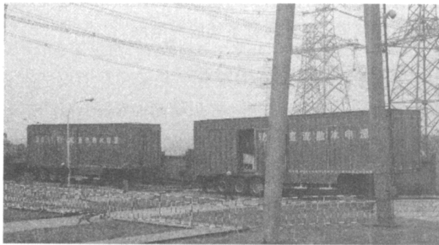
图7 直流融冰变电站试验现场 Fig.7 Experimental locale of transformer substation for DC deicing
