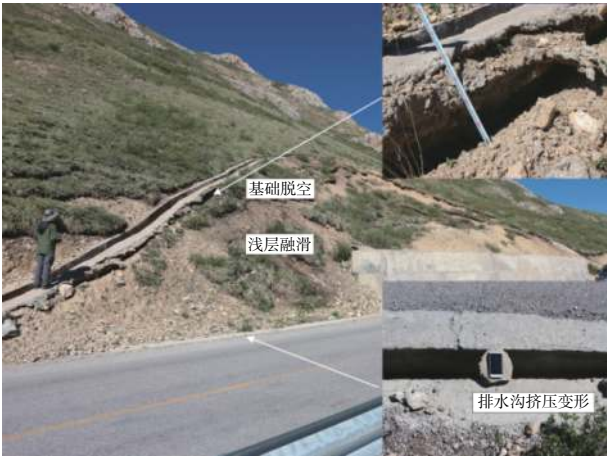
图 7 热融滑塌对排水沟的破坏照片 Fig. 7 Damage caused by hot melt slump
