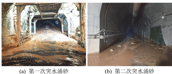
图2 小扑2#支洞 YX6+595.2 工作面突水涌砂灾害照片 Fig.2 Water and sand inrush disaster photos of YX6 + 595.2 working face in Xiaopu #2 branch tunnel
