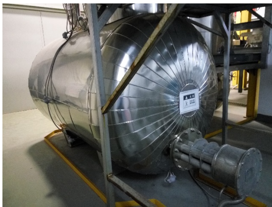
图3 熔盐储罐 Fig.3 Molten salt storage tank.
